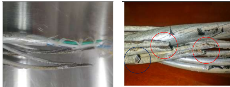
Figure 4. Left: failed section; right: fracture and material melting zone. Marked in red, sharp points can be observed
