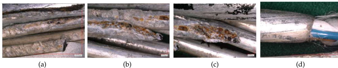
Figure 5. Affected area of the wires: a) oxidation and loss of material, b) loss of aluminum coating, c) oxidation and pitting of the coating as well as material loss, d) core tubing failure due to mechanical stress
