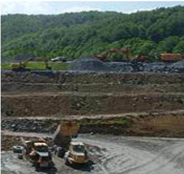
Figure 5. Unfinished works (Obras, 2017).
