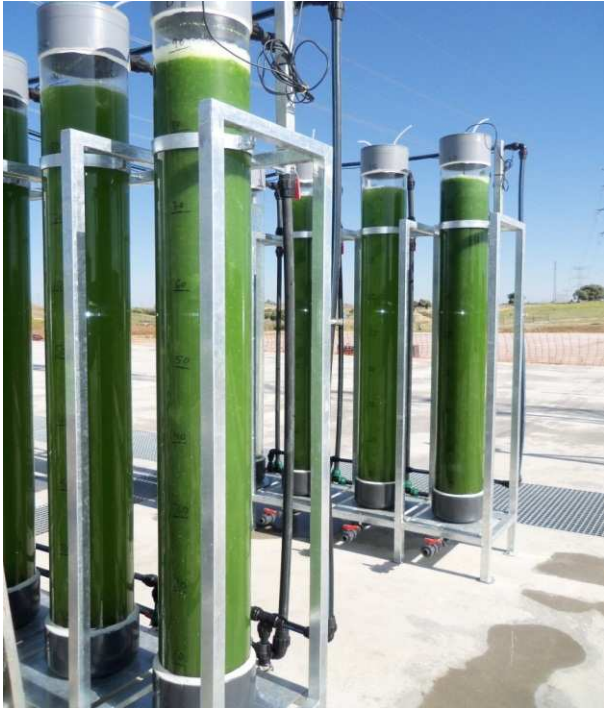
Figure 2. Algae treatment plant (Argos, 2017).
