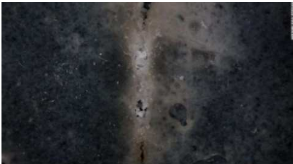
Figure 12. Crack in the concrete, 56 days after the action of the bacteria (Alvarez, 2017).
