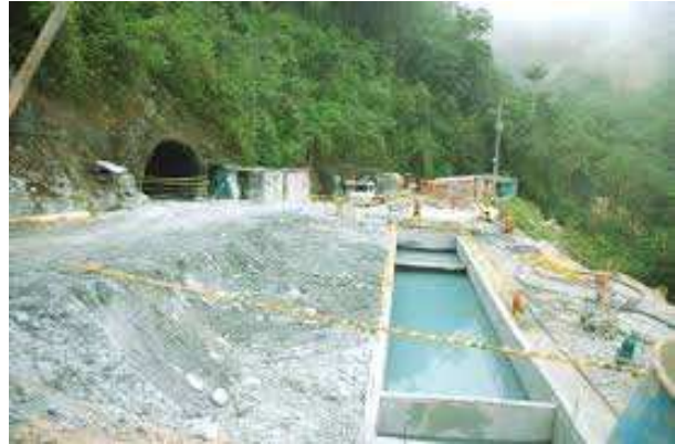
Figure 9. Water pollution from the construction site (Cronica del Quindío, 2017).
