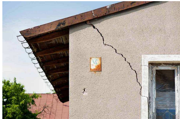
Figure 2. Earthquake-induced cracks (WebAdictos, 2017).
