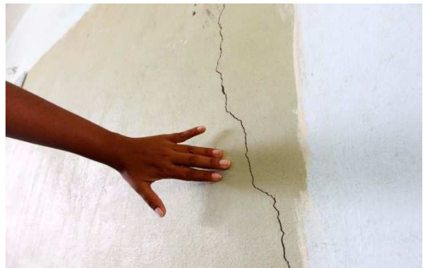
Figure 6. Cracks in the wall (Ayala, 2017).
