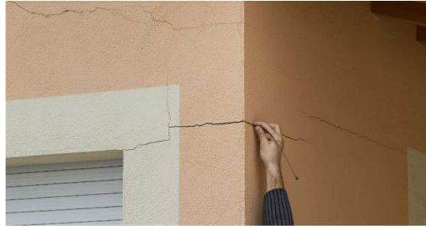
Figure 1. Crack in the house (Gonzalez, 2017).
