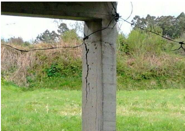
Figure 8. The PSOE denounces that the columns of the laundry have cracks (Arteixo, 2014).
