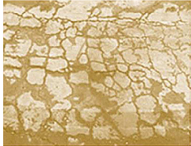
Figure 2. Asphalt layer without recycled rubber mix.
