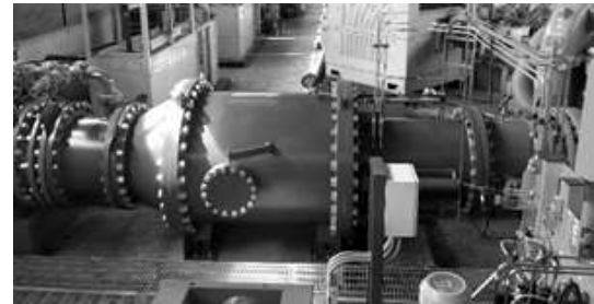
Figure 16. Multijet valve for turbine bypass. Source: own.
