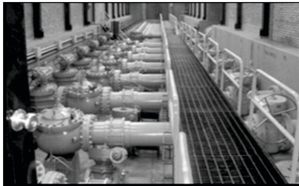
Figure 4. Usaquén PRS Valves [21].
