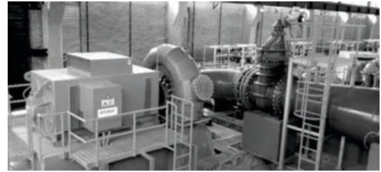
Figure 15. Gate valve and discharge pipe. Source: own.
