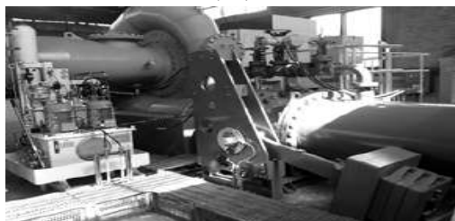
Figure 14. Admission pipe and butterfly valve. Source: own.
