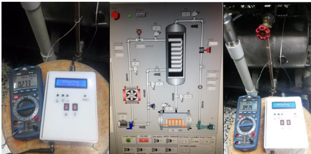
Figure 21. Measurements in the thermal plant.
