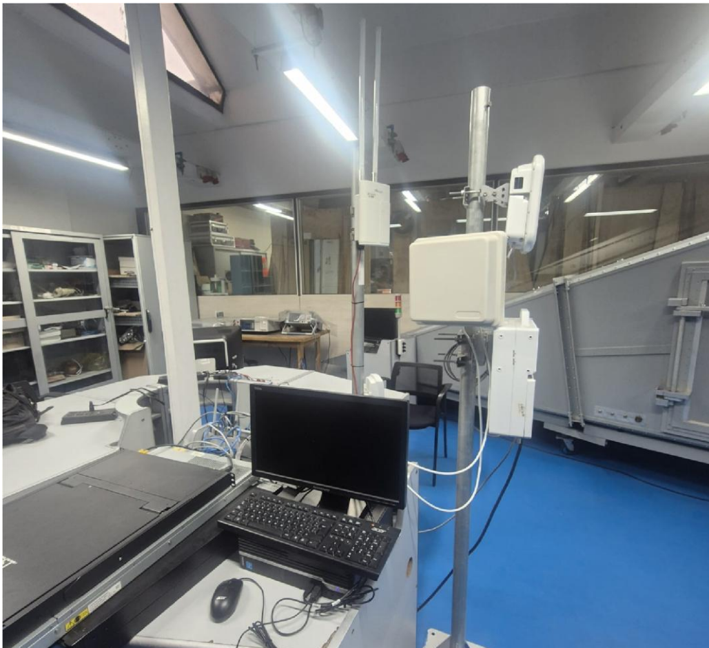
Figure 6. Our infrastructure for cellular networks.
